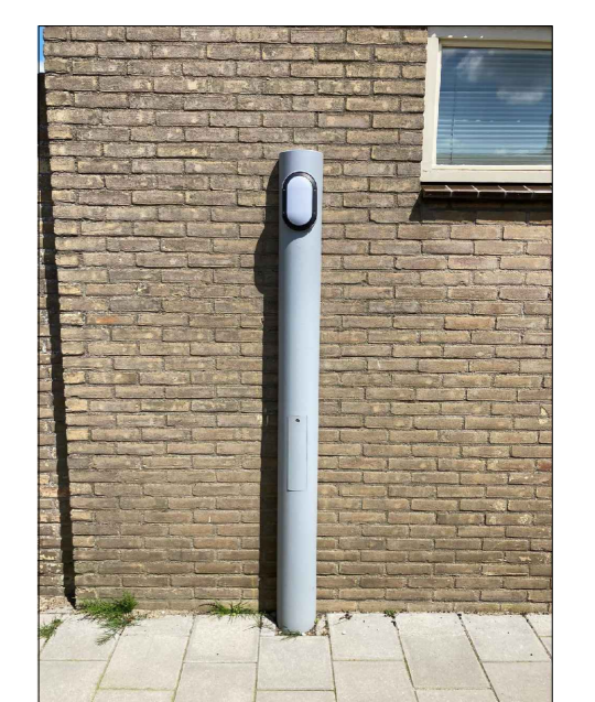
LICHTMAST TYPE BRANDLIGHT
